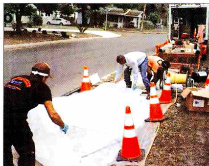
Using spot repair, crews are able to work in a small site area and reduce disruption associated with open-cut.
