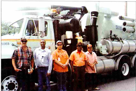
Lakeland, Fla., city crews, from the left Drew Adcock, Horace Taylor, Thomas Bryson, George Bennefield and Nelson Ramirez, have been completing spot repairs since May 2000.
