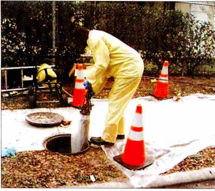
After cleaning and inspecting the pipe, the liners are lowered into a manhole and pulled into place.
